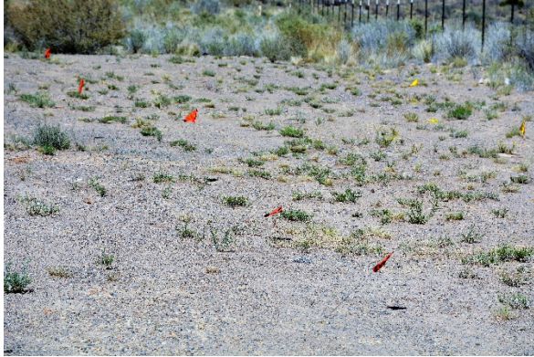
Utility flags mark the way for digging to begin soon for the new UNM-Gallup sign.
